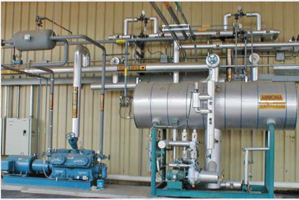
Ammonia Compressor and Pump System
