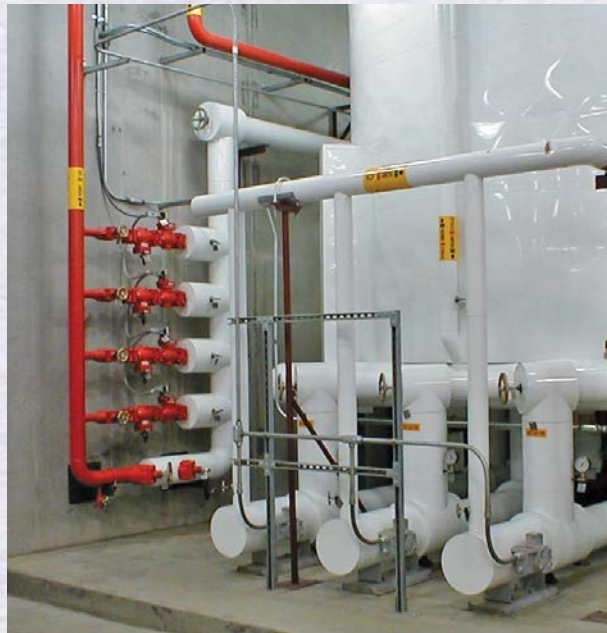
Ammonia System Recirculator
