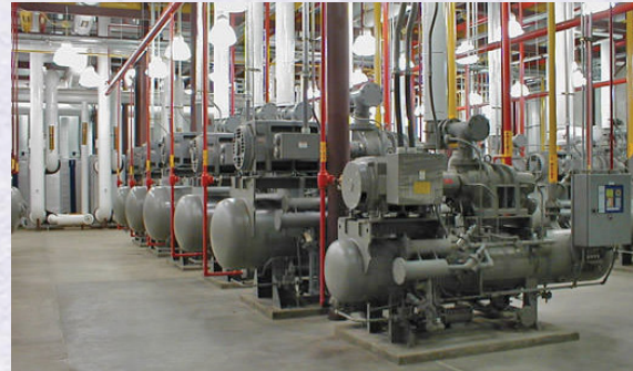
Ammonia System Machinery
